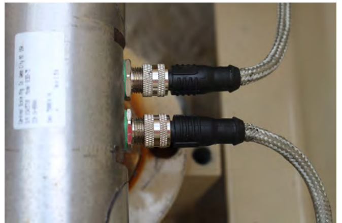
Install the load cell cable connectors on the load cell fittings and hand-tighten.
